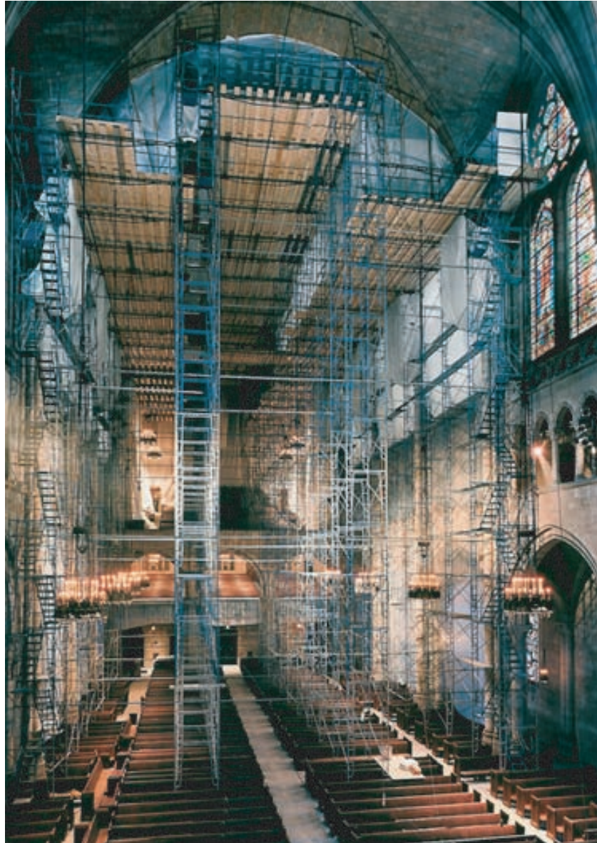
Photo: Urban D.C. erected a nine-storey scaffolding inside the sanctuary to clean and repair the Guastavino ceiling and make the necessary acoustical improvements.
