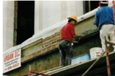
Photo top: Completed full restoration. Photo bottom left: Aerial view of the 40 x 60 glass atrium. Photo bottom right: Preparing the facade for installation of pre-cast stone ornaments
